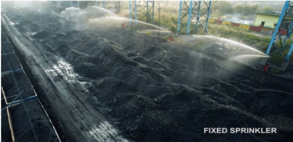
Fixed Sprinklers at Wharfwall
